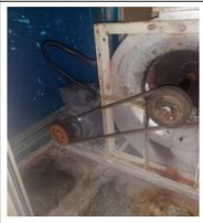
Photo name: Fan center checked normal date: 2024.08.01.-08.24
