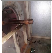
Photo name: Fan center bearing changed date: 2024.08.01.-08.24
